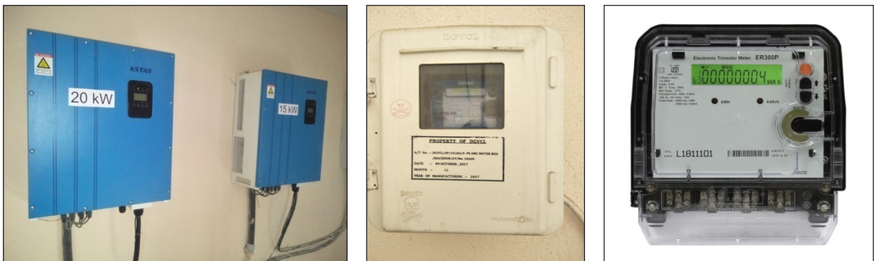
Fig. 5. 20 kW and 15 kW DC/AC 3-phase inverters, solar meter and bi-directional meter.
