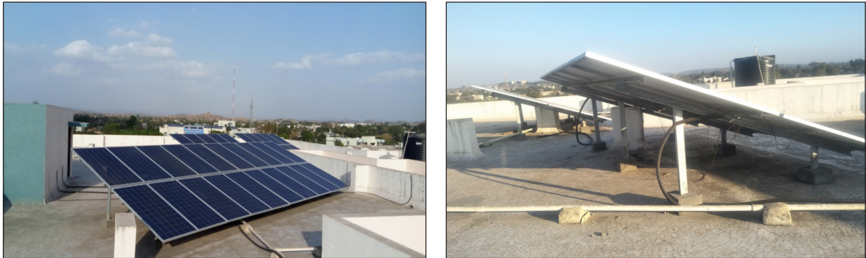
Fig. 4. 35.2 kWp rooftop grid interactive solar PV system and GI supporting structures with concrete pillars.
