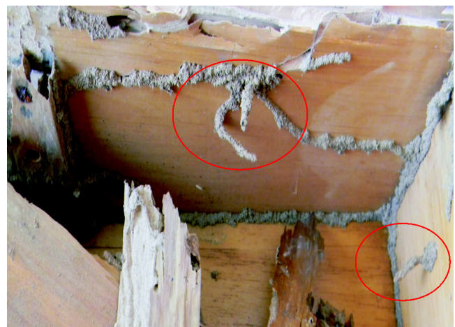
Fig. 2 Termite infested wooden box (characteristic hanging mud tubes)
