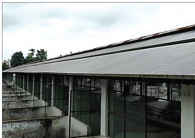
Fig. 3. Solar panels on roof can reduce temperature inside pig house and generate electricity
