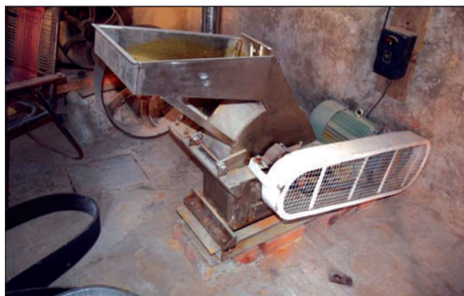
Installed pulverizer under FFP
