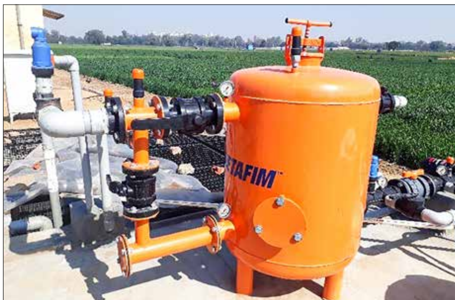
Drip irrigation system
