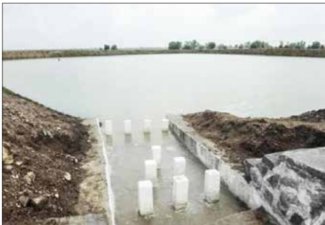
Farm pond with chute inlet spillway in Parbhani, Maharashtra
