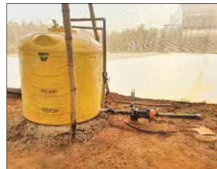
Developed three stage fertigation system Source: AICRP-PEASEM, Dapoli
