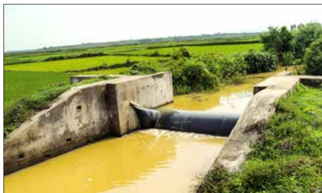
A flexi check dam across the water stream (water flowing over inflated rubber)
