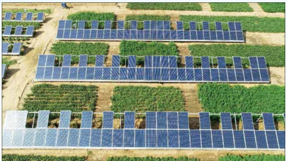
Ground mounted Agrivoltaic system at ICAR-CAZRI, Jodhpur
