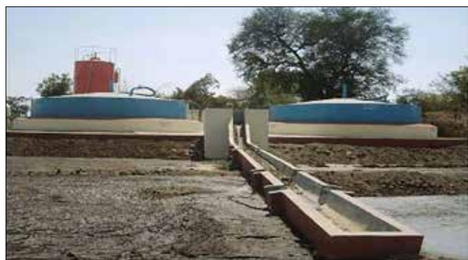
Community biogas plant at Bhintbudrak Distt. Surat, Gujarat
