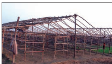
Fig. 4. Four-rack arrangement in a shed
