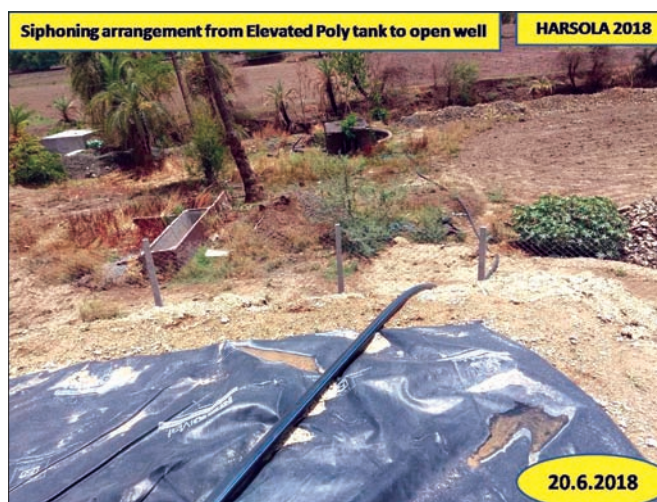
Fig. 2.b. Siphoning from storage tank to open well
