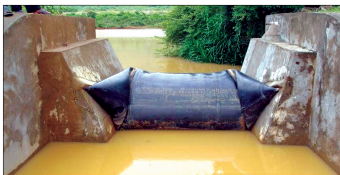
Fig. 2. Multipurpose rubber dam for watershed
