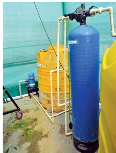
Water softener and collection tanks
