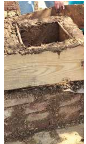
4. Complete filling the frame with a mixture of cow dung, straw, clay, and water
