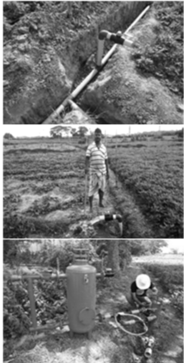
Photo 1. Pipe conveyance system in the canal command
